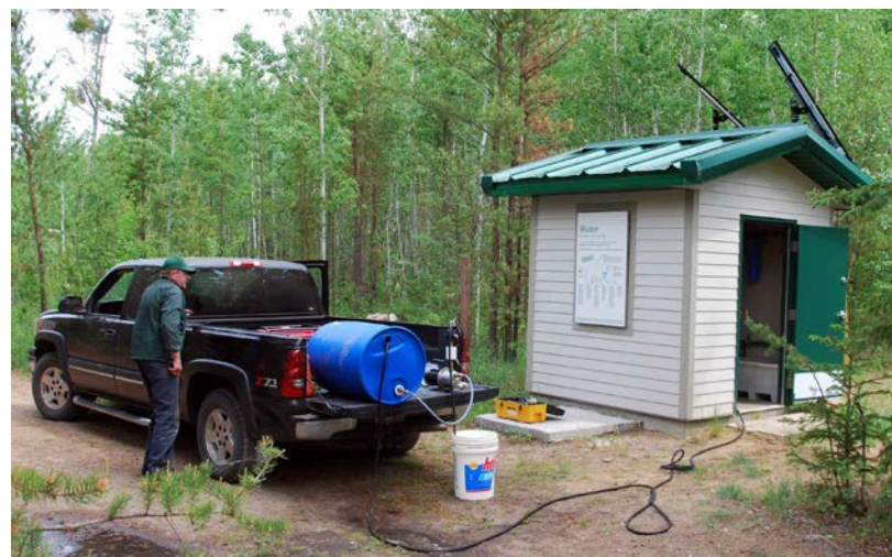
Figure 1. Field sampling at the solar powered pumphouse at First Mustus Lake. Raw well water was pumped into the barrel and then re-pumped through the Filta-Max filter.
